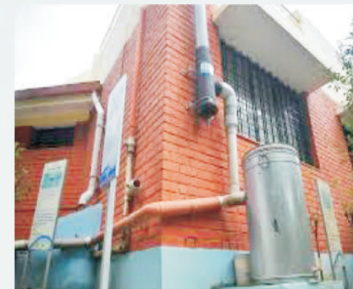
Rain water harvesting system
